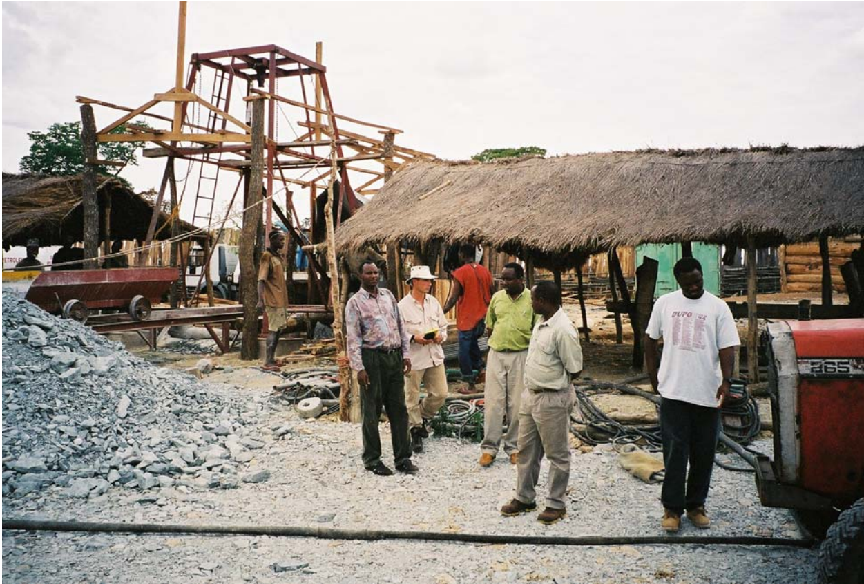
Plate 1. View of pit head and waste rock tip, Blue Reef Mine, Rwamagasa
