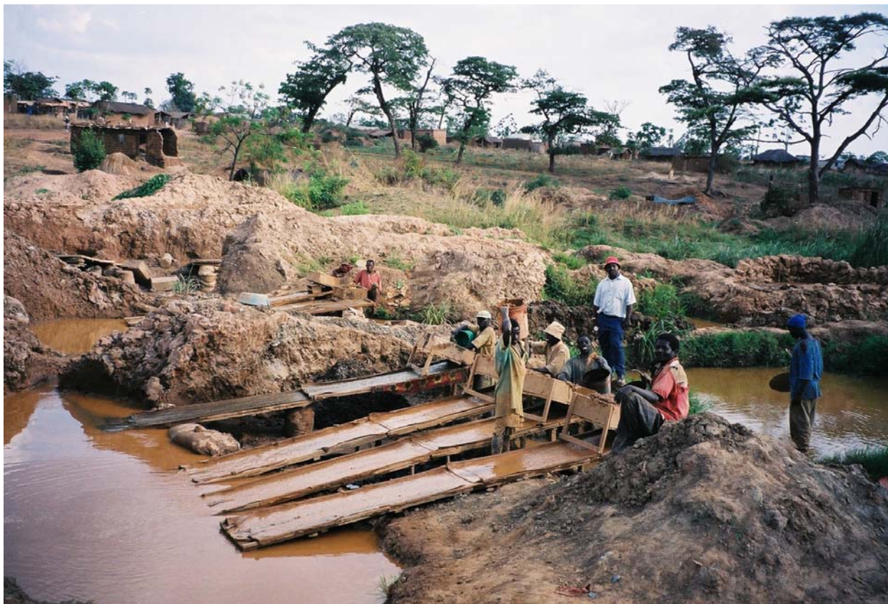
Plate 18. Sluices at tailings reprocessing site (A42-43) on the slope to the north of Rwamagasa village.
