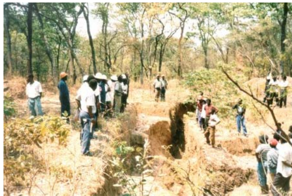
Dangerous excavation in Ndola Rural mines
