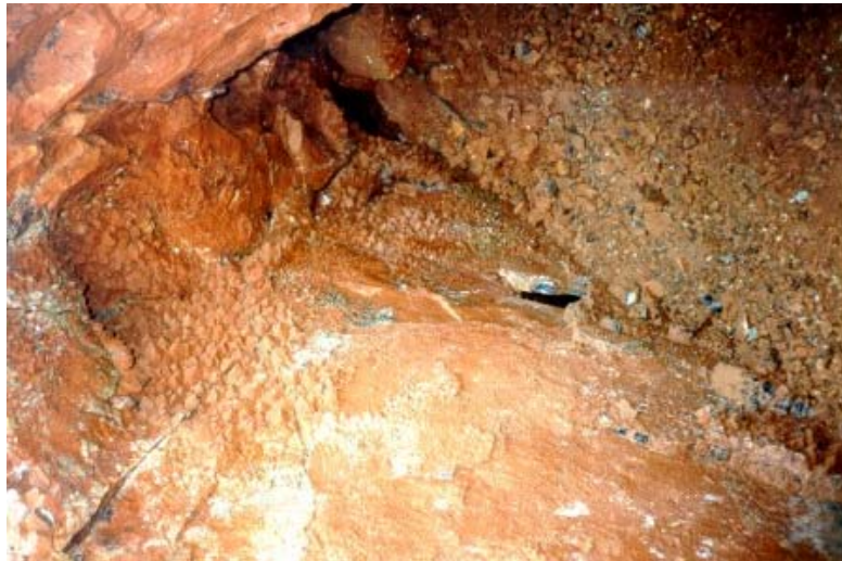
Safety hazard posed by mining excavations in Kalomo mining area
